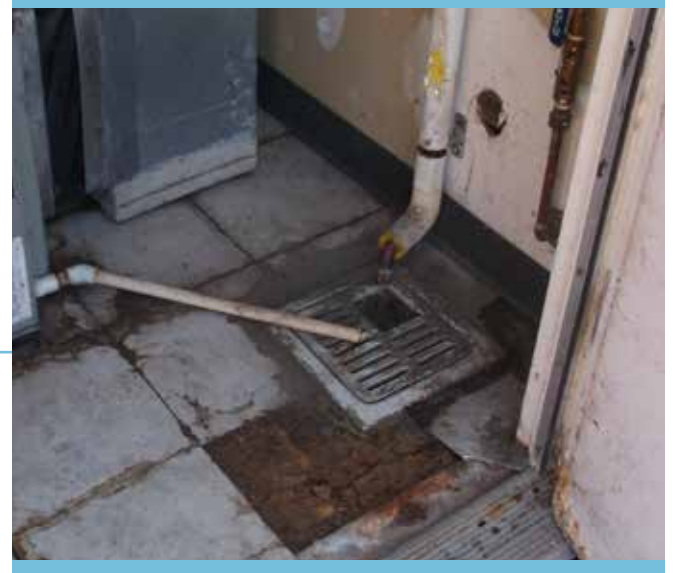
HVAC Room at Shoal Creek Elementary School
